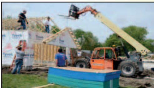
Men of Grace UMC in Naperville use a mobile crane to raise a gable at a Fox Valley Habitat for Humanity house. Photo by Al Benson.
