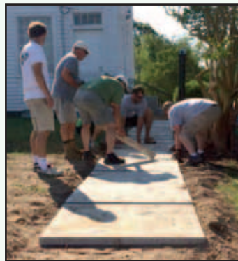
Volunteers join Jarrett in building a walkway to a church building that served as the Trinity home until a new building was constructed in 1954.
